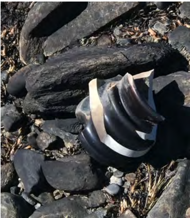
Broken insulator located on the ground near pole 40456 (old pole number 17406).
