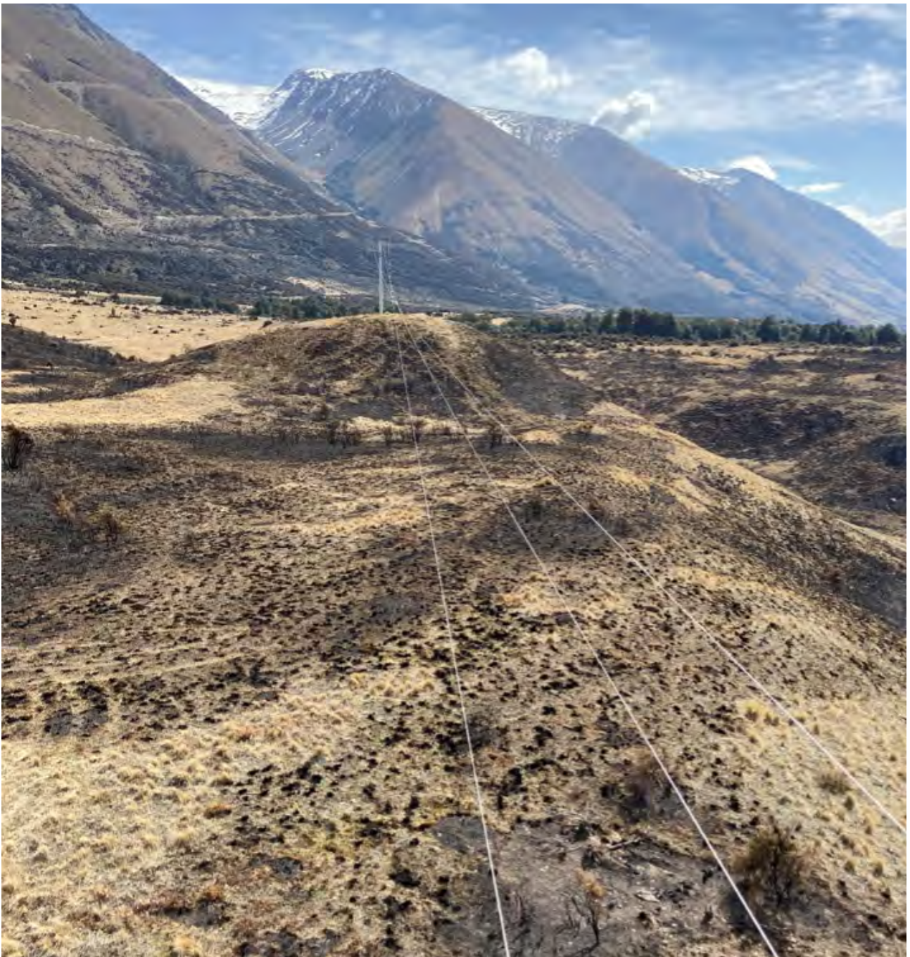
Span between Pole 35693 and Pole 870452 showing the twist in the lines.
