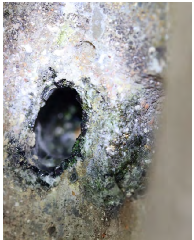
Arc damage on pole 35693.
