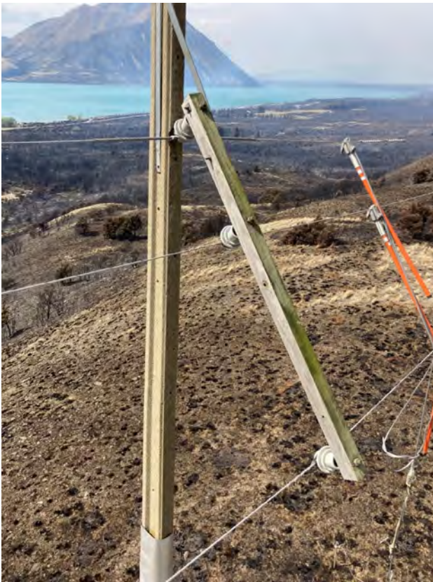
Pole 35693 with the cross-arm rotated over.
