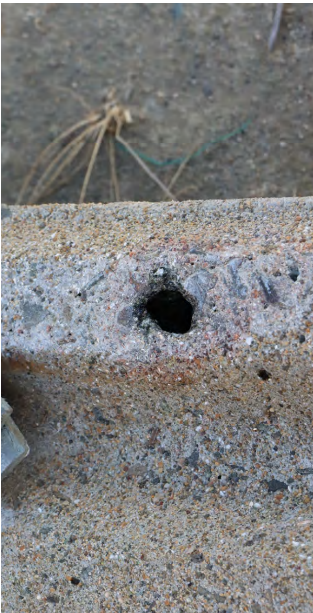
Close up of the burn hole on pole 35693 below the centre bolt holding the metal stay arms to the pole. It has been exposed to intense heat.
