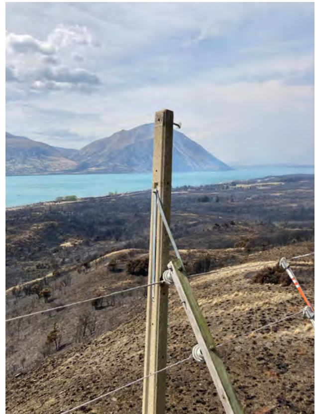
Pole 35693 showing the lakeside metal stay arm hanging in the centre of the pole and the centre bolt that secured the wooden cross-arm to the pole has moved backwards but remains in the pole (note bolts have a single nut).
