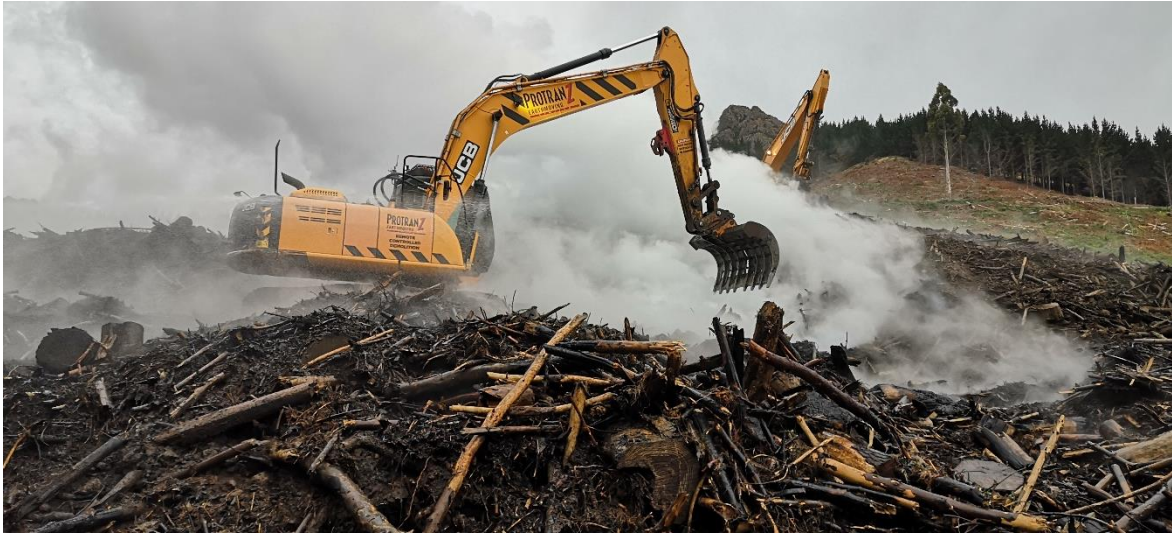
Image 2. Example of an excavator with root rake (B. Janes, FENZ. Packhorse Hut, Gebbies Pass).
