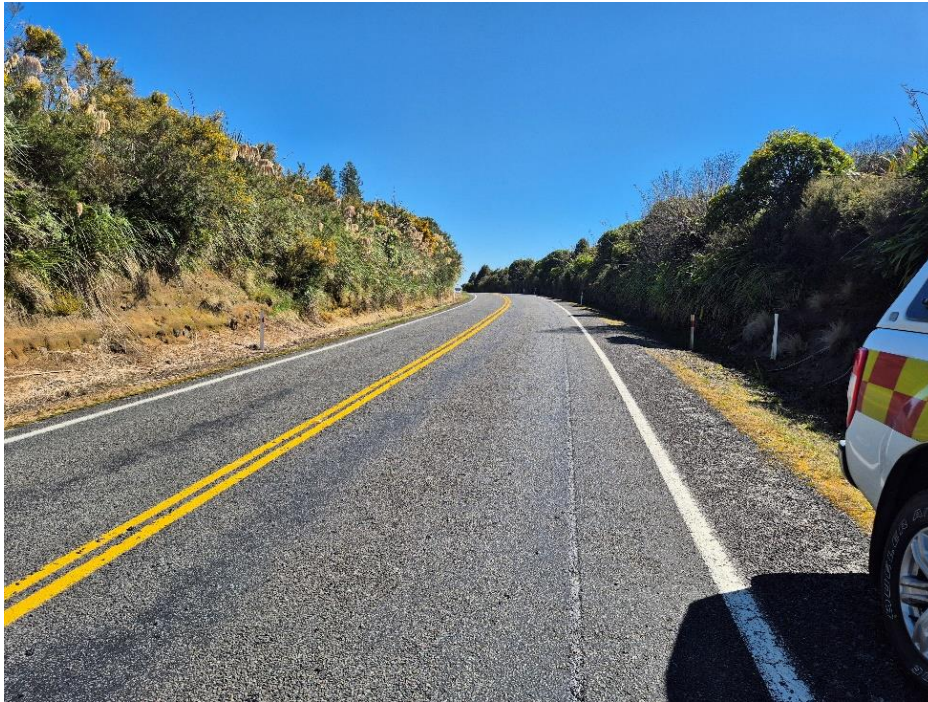
Figure 4. and 5. Road damage caused by broken trailer axle
