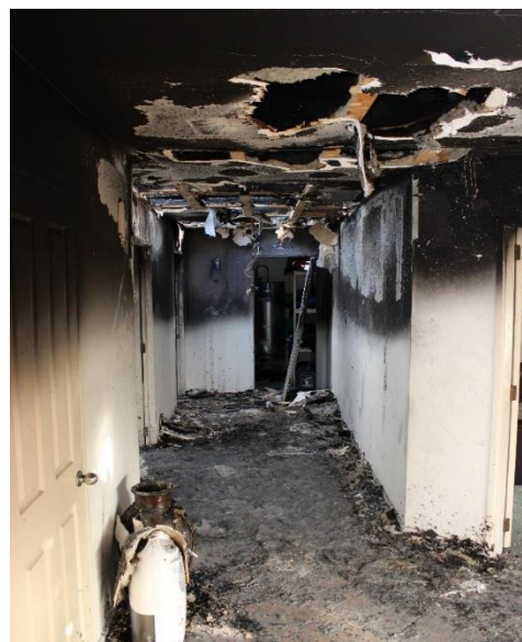
Photo above shows extensive fire damage in first unit.
