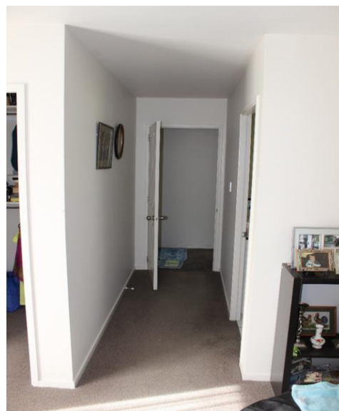
Photo below shows undamaged adjoining unit in same house protected by a well constructed fire wall.
