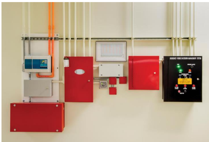
Figure 4 – Emergency generator supervisory panel
