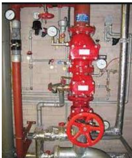
Figure 5 – Typical valve group arrangement with main stop valve prominent
