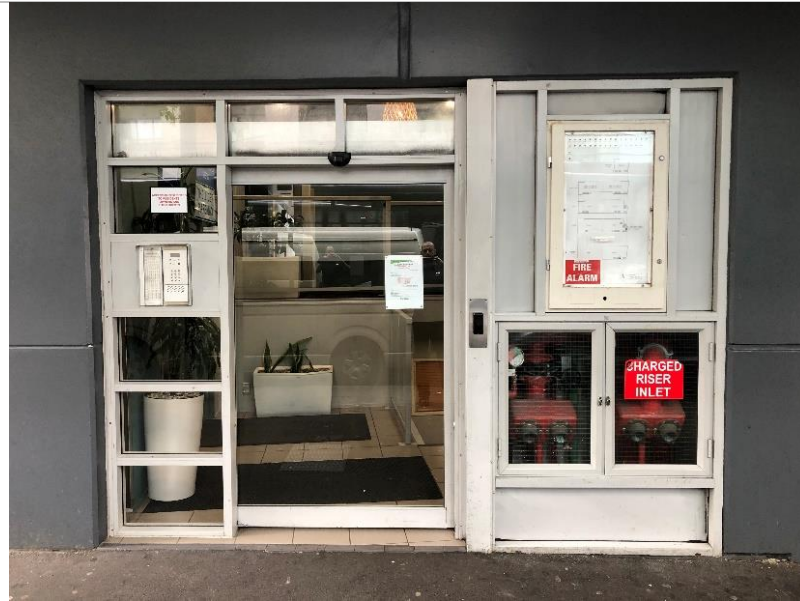
Figure 5 – Panel and facilities co-located at entry point
